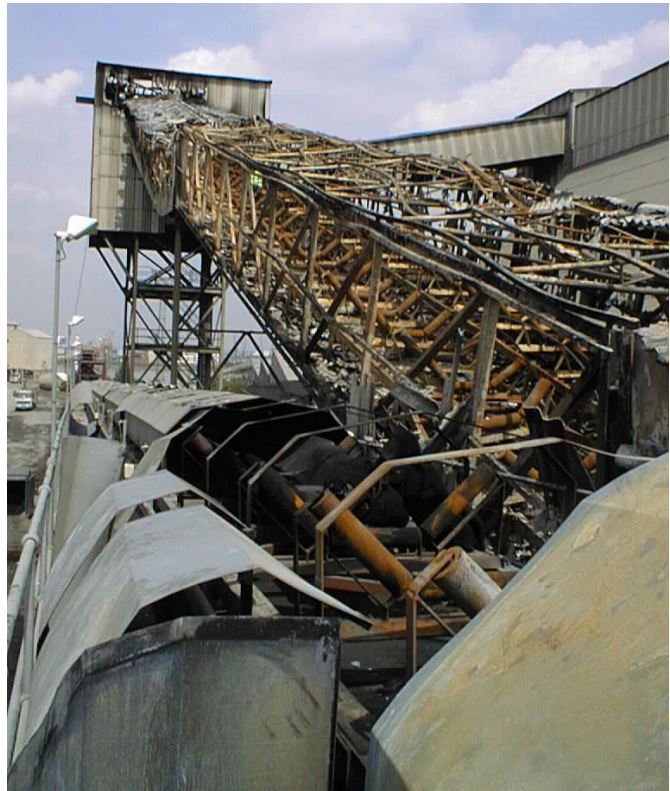
Figure 5. A blazing belt spreads fire very quickly.
