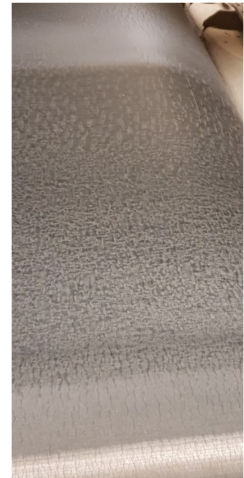
Close up of ozone cracked belt
