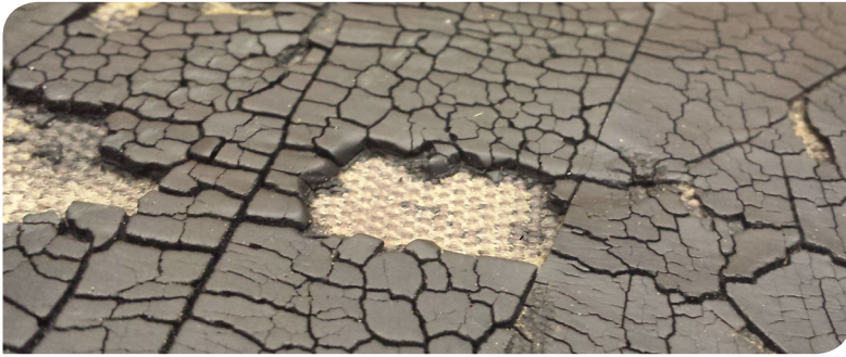
Above: Severe wear caused by heat damage that has been accelerated by UV exposure.
