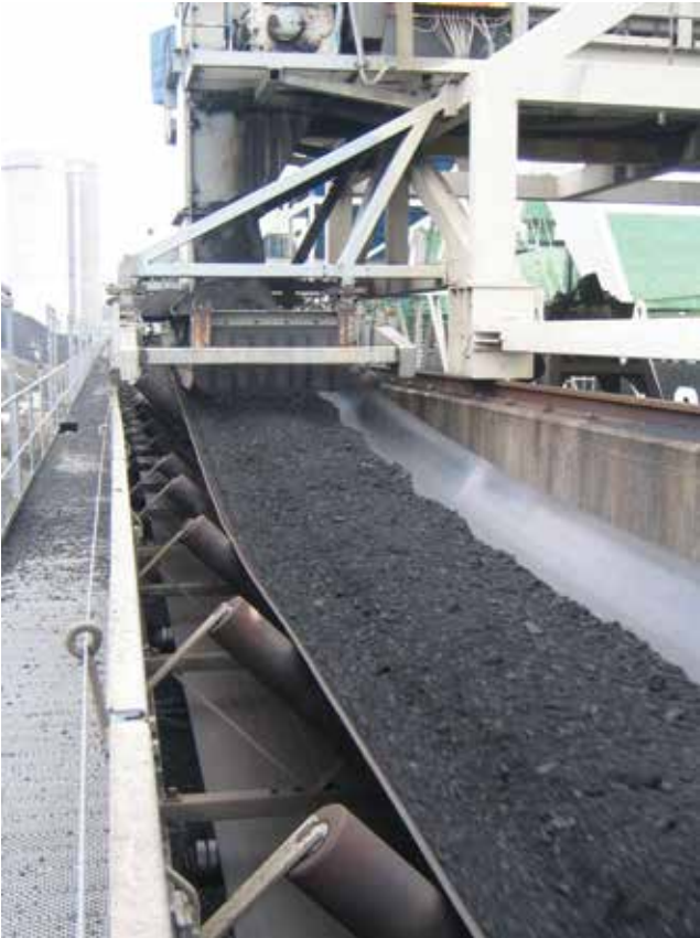
Conveyor belts are surprisingly complex technical components.
