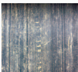
The first signs — small cracks appear in the surface of the rubber.
