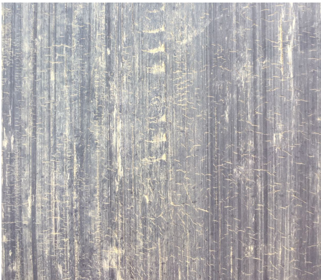
Figure 1. Ozone cracks in the surface of the rubber.
