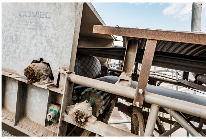
Figure 4. Transversal cracks deepen under the repeated stress of passing over the pulleys and drums.
