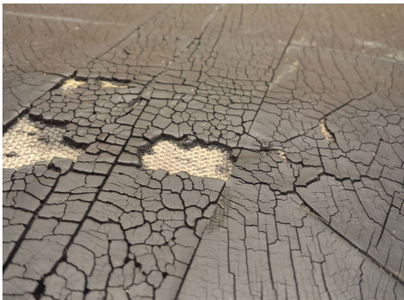
Any period longer than a few minutes at excess temperatures can cause irreparable damage.
