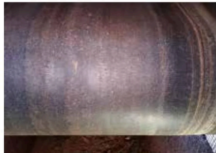
Cracking up – the result of rubber not having inbuilt protection against ozone and ultraviolet light
