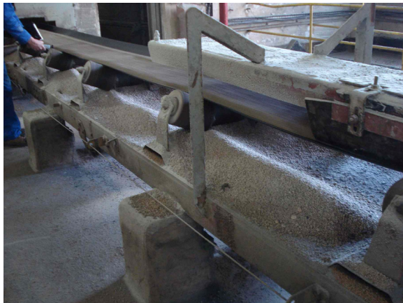
An unclean working environment is often the cause of accelerated wear and damage.
