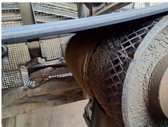
Belt slippage caused by waste matter on the drum increases strain on the motor.
