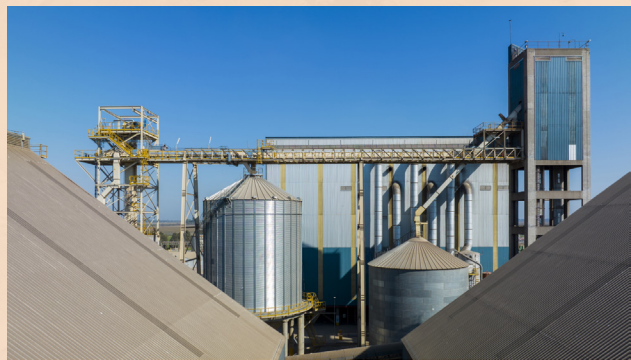
Figure 4. Bühler's enclosed belt conveyors at COFCO International's Timbúes facility, installed in 2023, Argentina. Image courtesy of Bühler.
