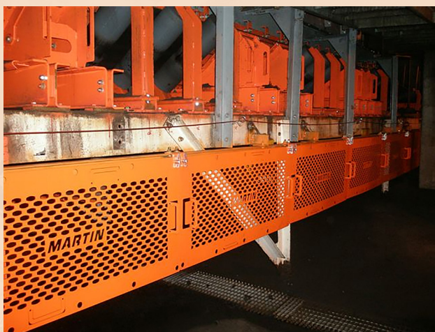
Figure 2. Redesigned loading zones for better loading, centring, and alignment. Image courtesy of Martin Engineering.
