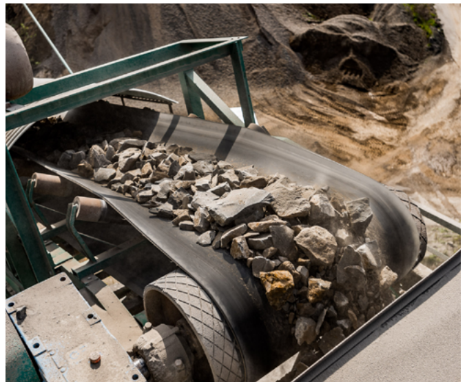
Misaligned drums and idlers cause extra wear.
