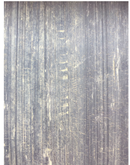
The beginning of the end – innocent-looking cracks in the surface of the rubber
