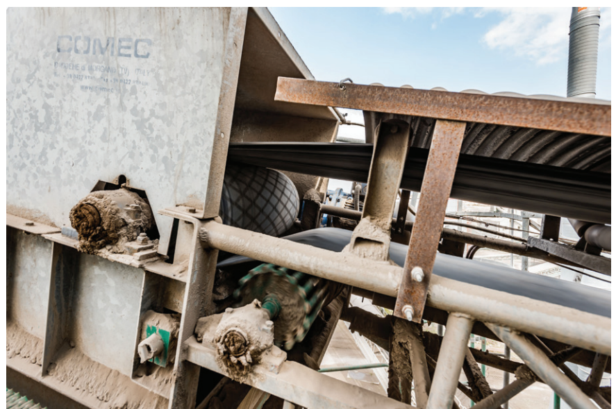
Transversal cracks deepen under the repeated stress of passing over the pulleys and drums
