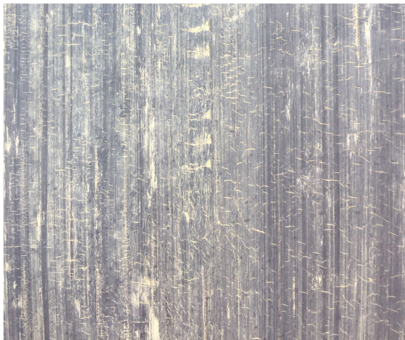
The beginning of the end. 'Innocent' looking ozone cracks in the surface of the rubber.
