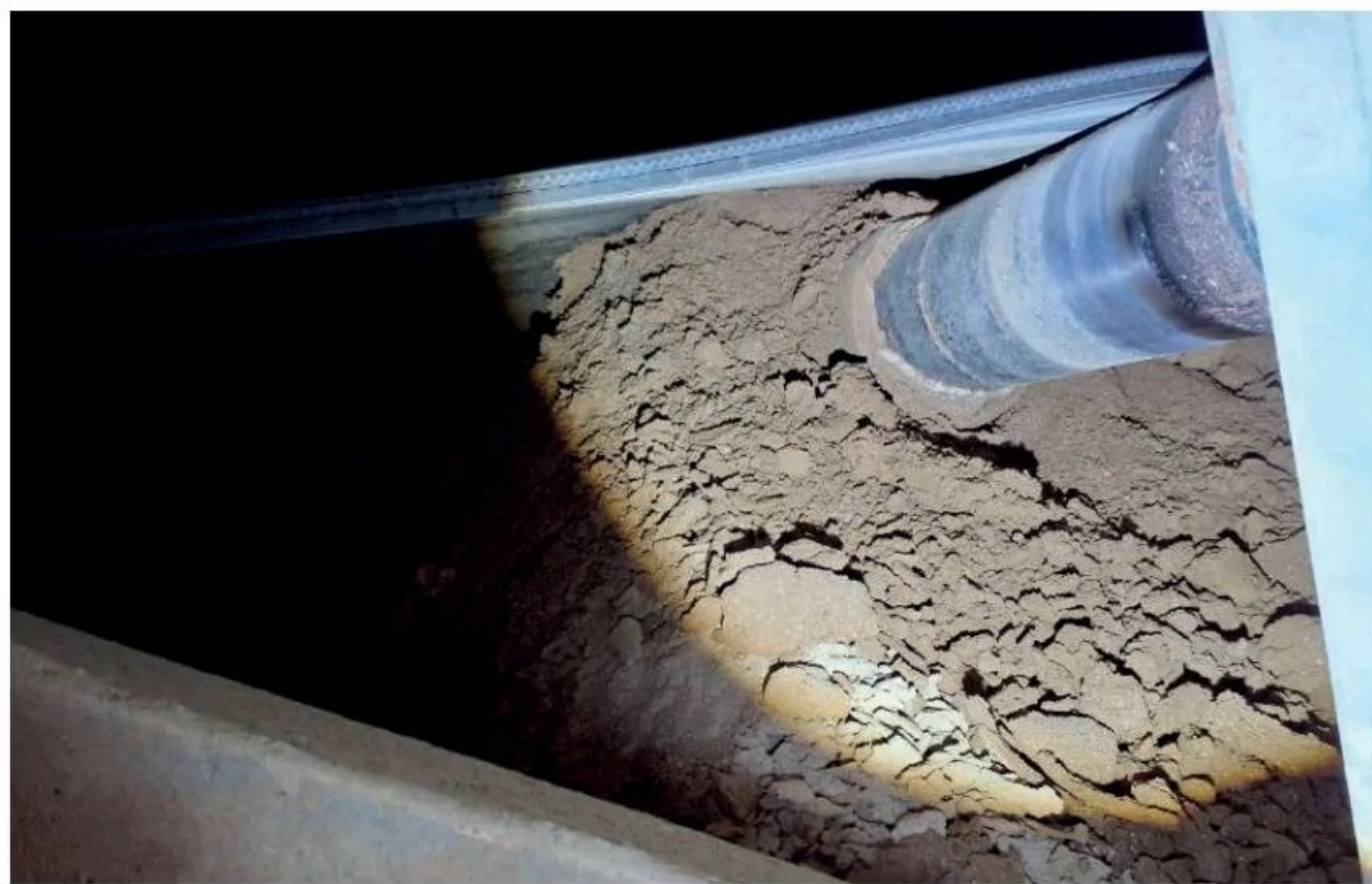
Figure 2. Unclean work environments are the most common cause of accelerated wear and damage.
