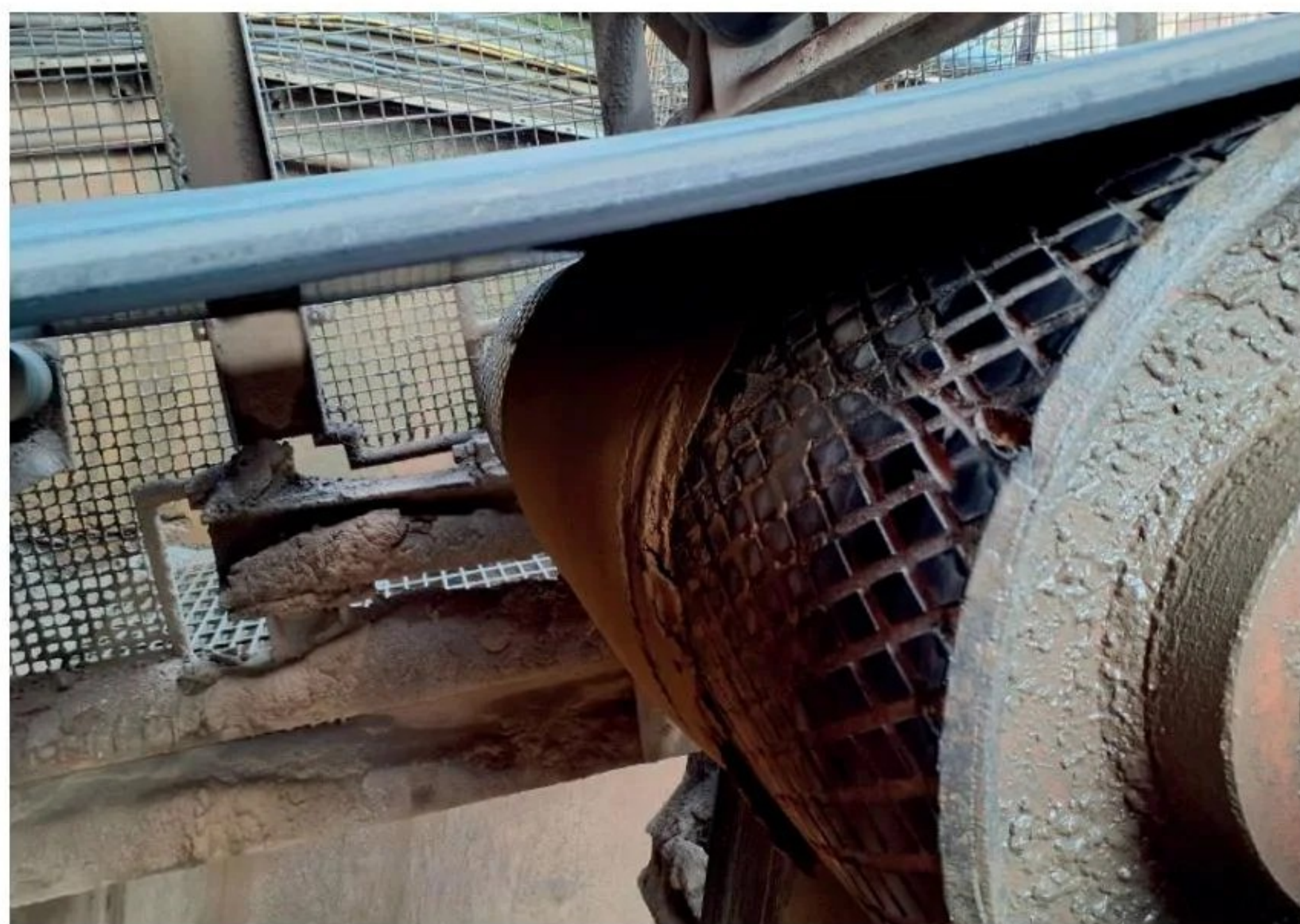
Figure 4. Belt slippage caused by waste matter increases strain on motor.
